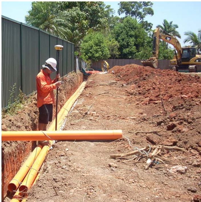
ABOVE: The team is busy preparing the project zone for major construction. Current work activities include finalising the relocation of existing underground services for telecommunications, power, water and sewage in local streets.
